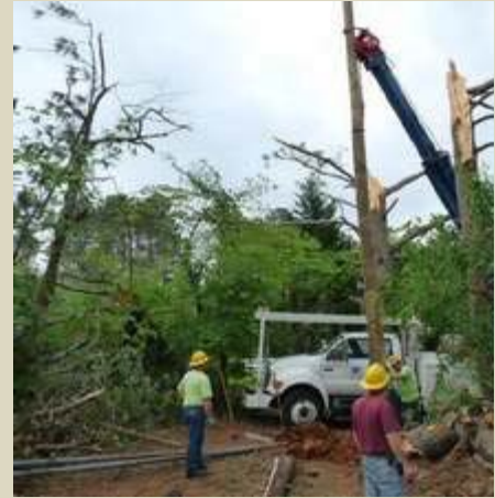
Richmond Power & Light workers set a power pole in an area just southeast of Chattanooga, Tenn. / Supplied photo Richmond Power & Light workers set a power pole in an area just southeast of Chattanooga, Tenn.
